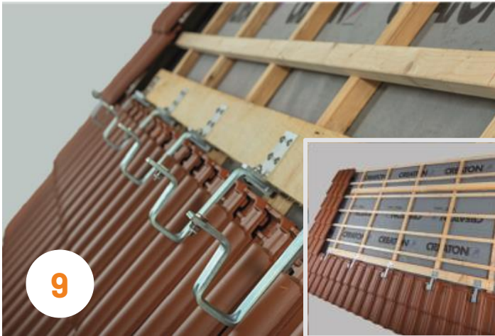
9 Screwing of all solar holders specified in the plan on the positioned wooden board. The specified center distances must be taken into account.
