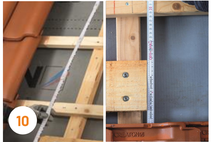
10 In accordance with the solar panel system, the board of the next row of supports must be prepared in the same way as previously showed.
