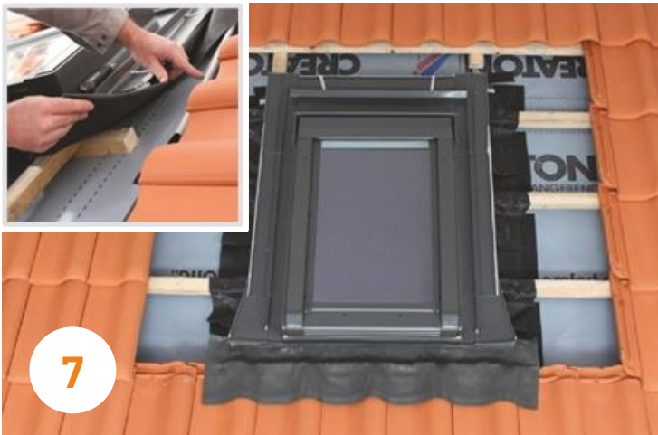
7 On the ridge side, the apron must be laid under the previously installed sloped gutter. Depending on the height of the roof tile profile, with low roof pitches it may be necessary to flatten the roof tiles in the upper area to such an extent that water can flow freely downwards.
