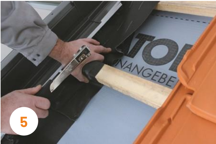
5 The vapor-permeable apron (Sd value 0.02 m) attached to the roof exit serves as a rainproof connection. It is placed tightly around the support battens and secured.
