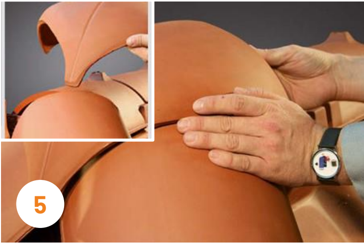
5 Position the hip cap tile onto the apex taking care not to leave too large a gap on any of the sides.
