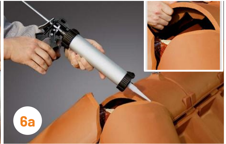
6a Mark the overlap of the hip cap tile on the hip/ridge tiles, then bond the three hip and ridge tiles to the hip cap using a high-quality adhesive (frost-resistant and suitable for ceramics)
