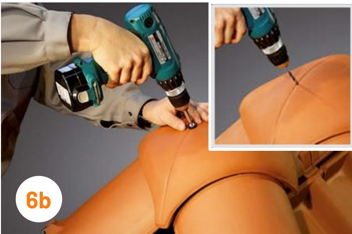
6b Drill a hole in the hip cap tile then fasten it to the timber structure below using a corrosion-proof sealing screw.
