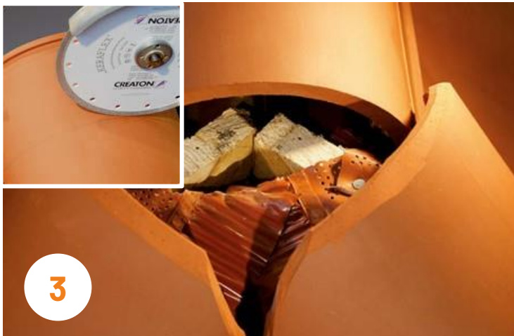
3 Cut and adjust the ridge and hip tiles in such a way that the hip cap tile is clearly supported at all three points
