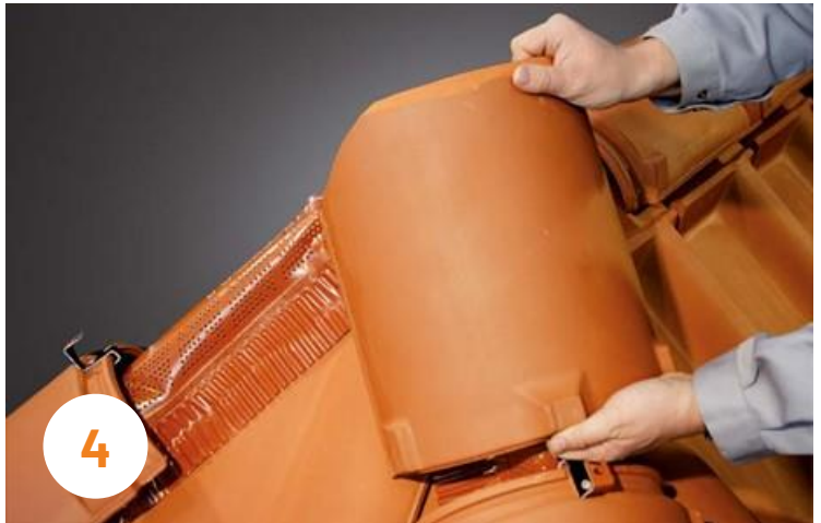
4 It is not necessary for the three tiles that meet at the apex to touch each other precisely. The hip cap tile has to overlap the three ridge tile by approx. 5-6 cm.
